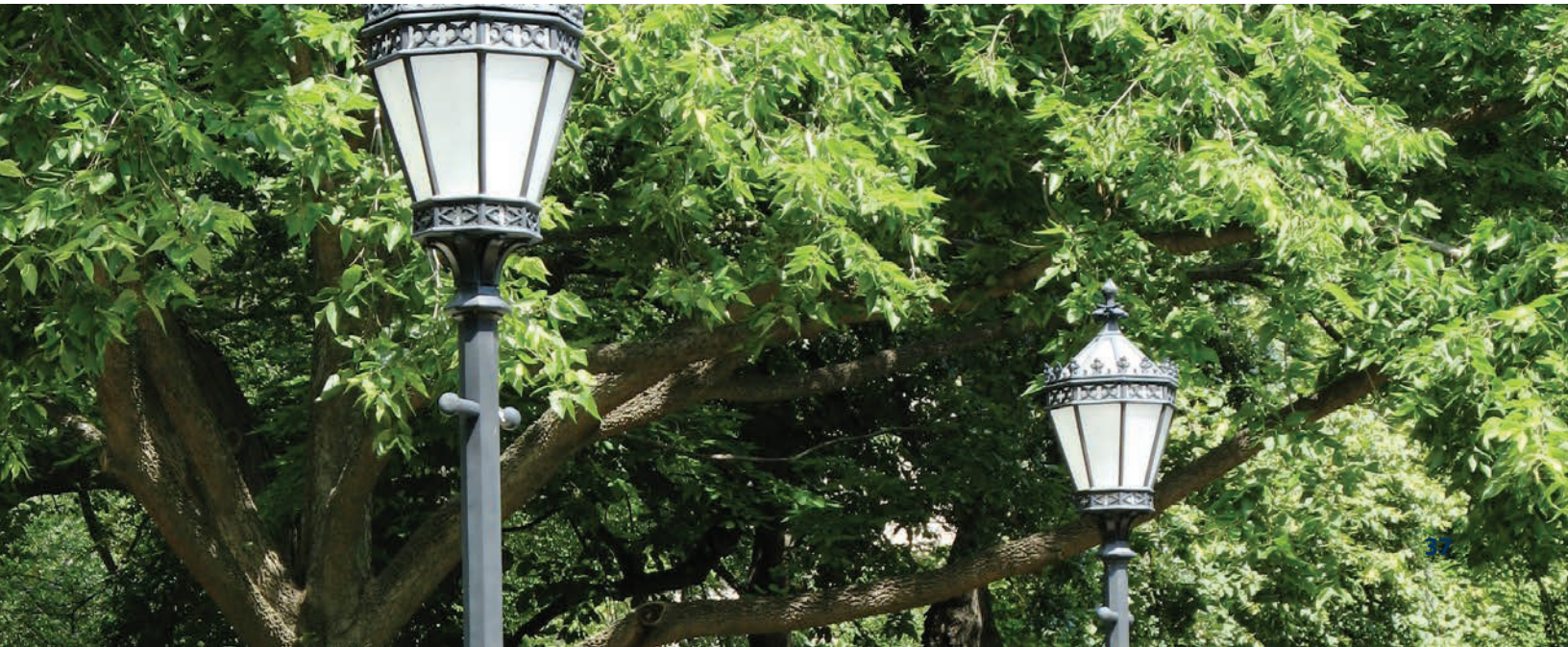
Stand-alone pedestrian lighting fixtures
